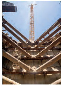
90-foot-deep access tunnels were dug to allow ingress into the freshly bored subway tubes.
